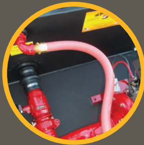
Fill-in connection with flexible hose
