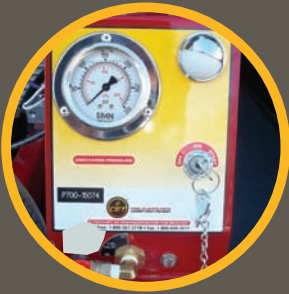
Control panel with master switch, light and pressure gauge
